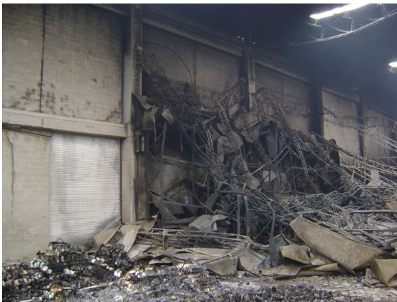
Figure 5. Varying degrees of damage
