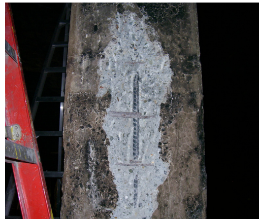
Figure 6. Assessment of fire damage with the concrete color
