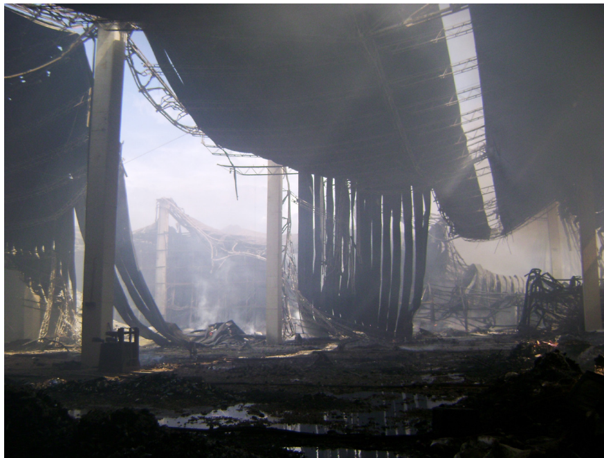
Figure 2. Warehouse after the fire
