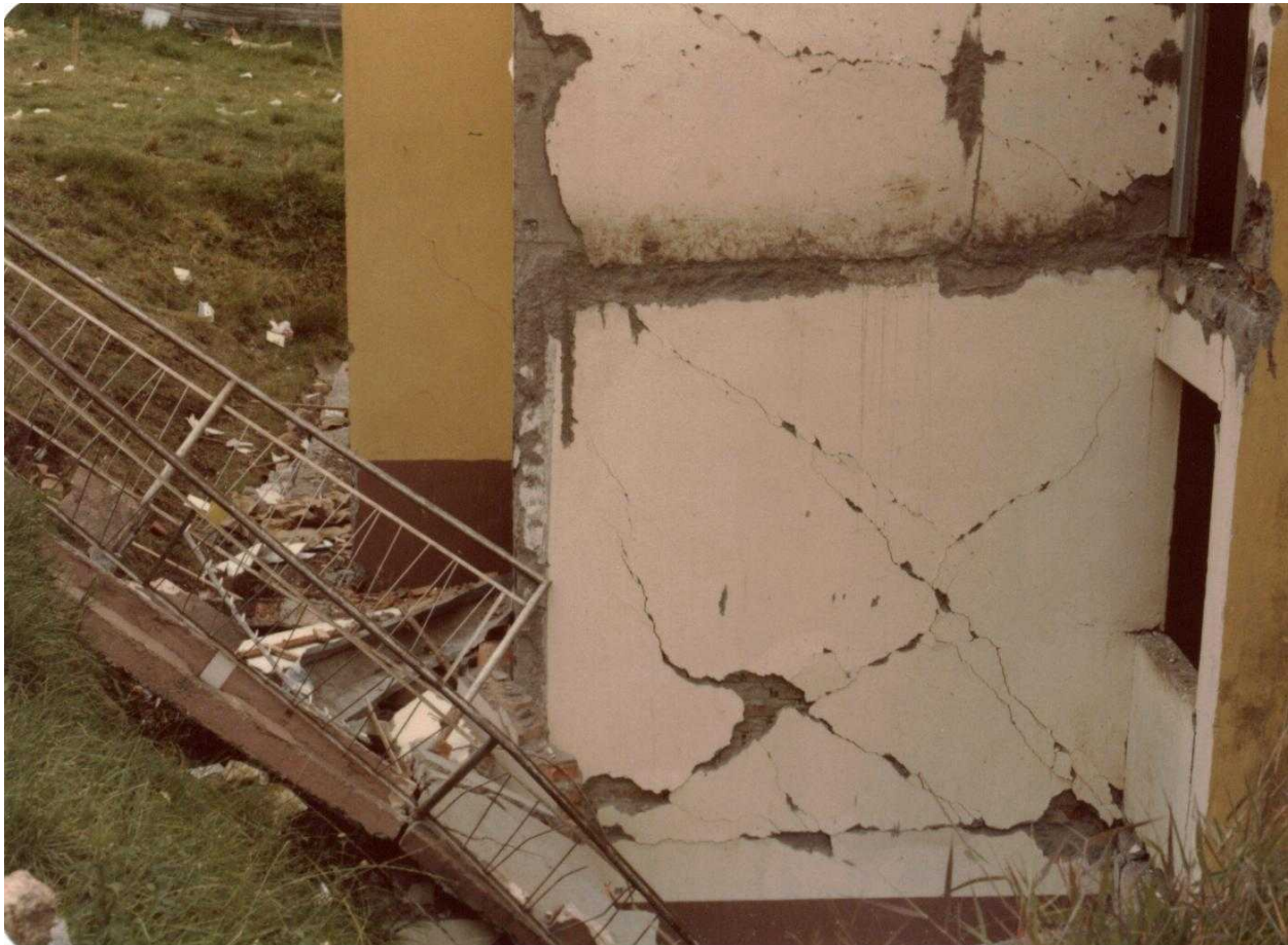
FIGURE 6H: Typical Earthquake Damage - Importance of the Details in Seismic Design : The "access bridge" to this building did not have adequate bearing length and had collapsed, thus leaving inhabitants without a means of escape
