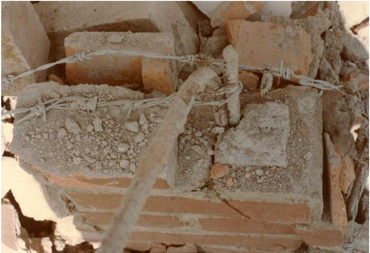
FIGURE 5F: Seismic Deficiencies - Poor Quality of Materials (mortar and grout); Inadequate Vertical and Horizontal Reinforcement.
