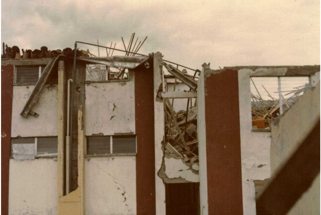
FIGURE 5B: Seismic Deficiencies - Discontinuous R/C Bond Beams.
