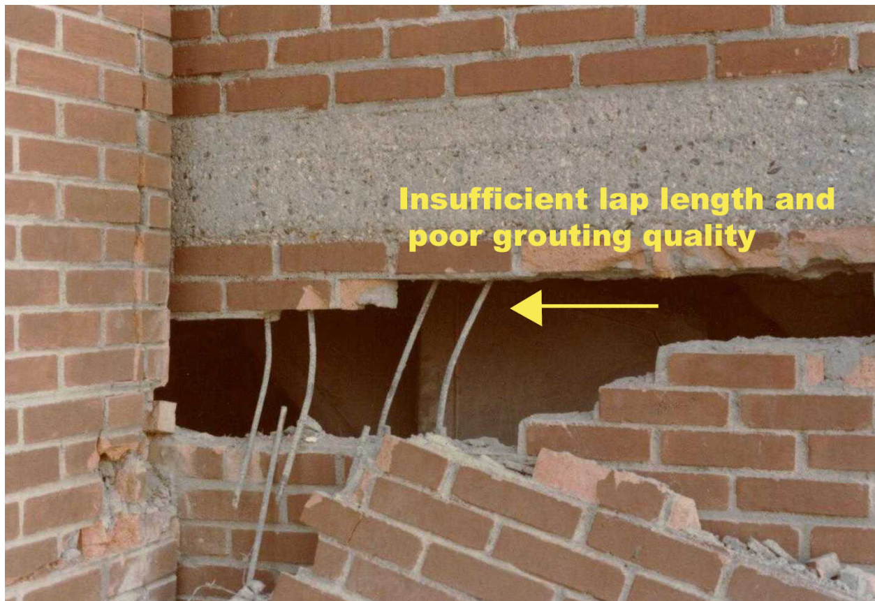
FIGURE 5A: Key Seismic Deficiencies - Inadequate Reinforcement and Poor Grouting (note the reinforcement bar slippage)
