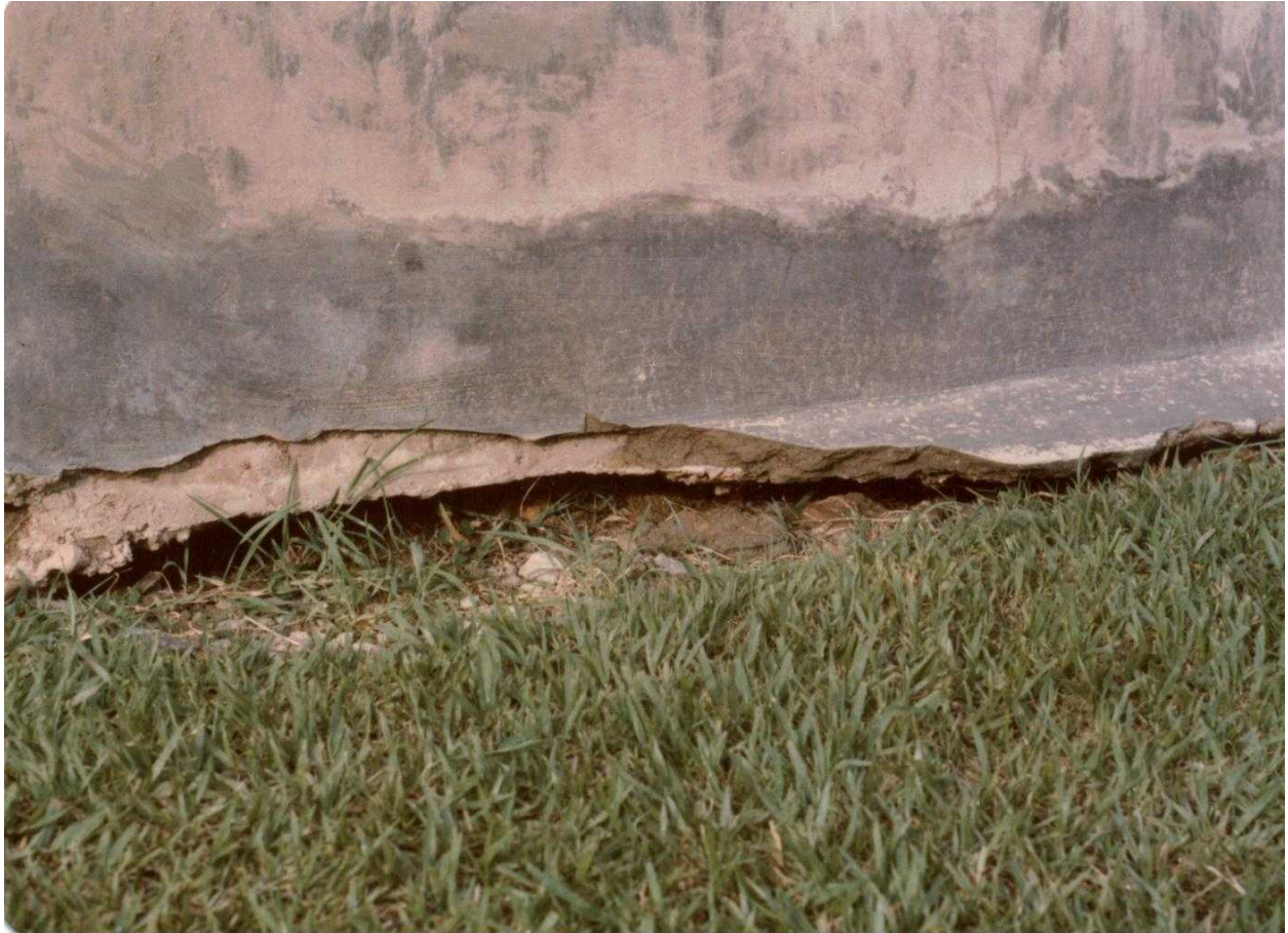
FIGURE 5H: A building weakened due to tilting induced by a pre-earthquake foundation settlement (separation between the two buildings was 100 mm at ground level but 0 mm at the top). Such buildings are likely to suffer more extensive earthquake damage.
