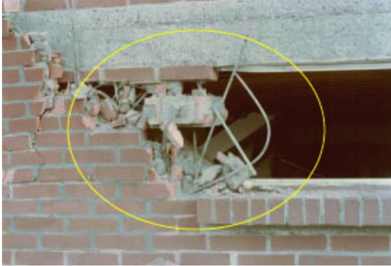
FIGURE 6B: Typical Earthquake Damage - Inadequate Reinforcement (Detail A shown on Figure 6)
