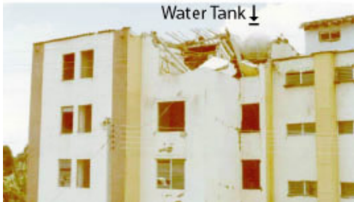
FIGURE 6G: Typical Earthquake Damage- Collapsed Roof; note the absence of continuous RC bond beam and the wall-roof connection; the water tank at the roof "walked off" and had contributed to the roof collapse.
