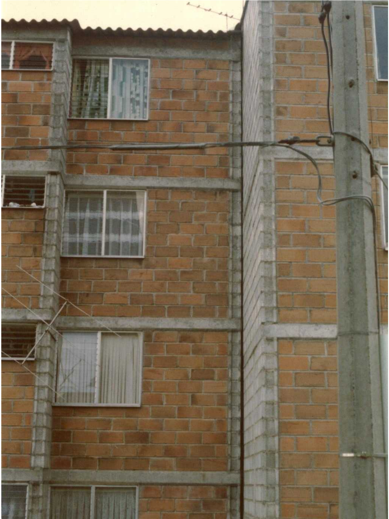
FIGURE 5G: A building weakened due to tilting induced by a pre-earthquake foundation settlement
