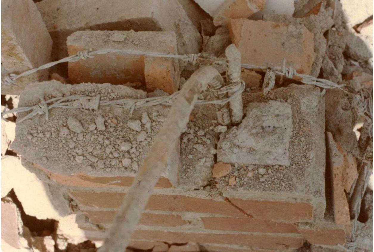
FIGURE 6E: Typical Earthquake Damage - Poor Workmanship and Inadequate Reinforcement (this is an enlarged detail B shown of Figure 6c)
