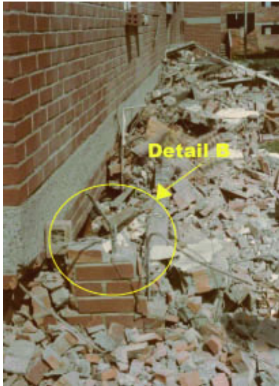
FIGURE 6D: Typical Earthquake Damage - Detail B Shown on Figure 6b
