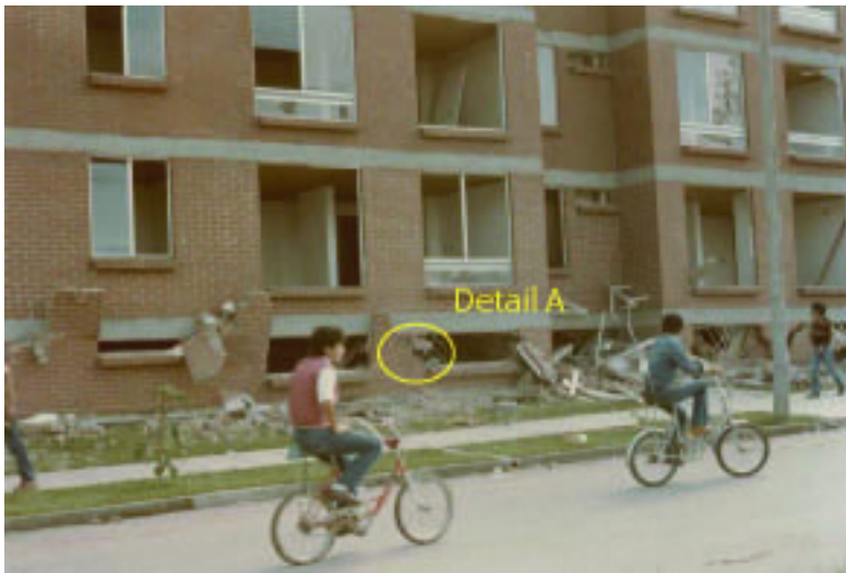
FIGURE 6A: Typical Earthquake Damage- Failure of Load bearing Masonry Walls
