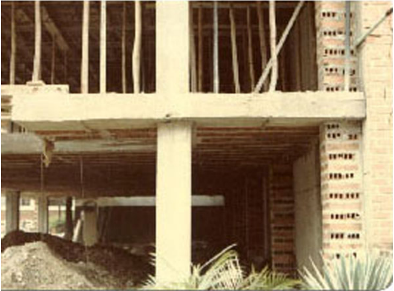
FIGURE 5D: Poor Design - Combination of Concrete Frames and Unreinforced Masonry Walls or Pilasters
