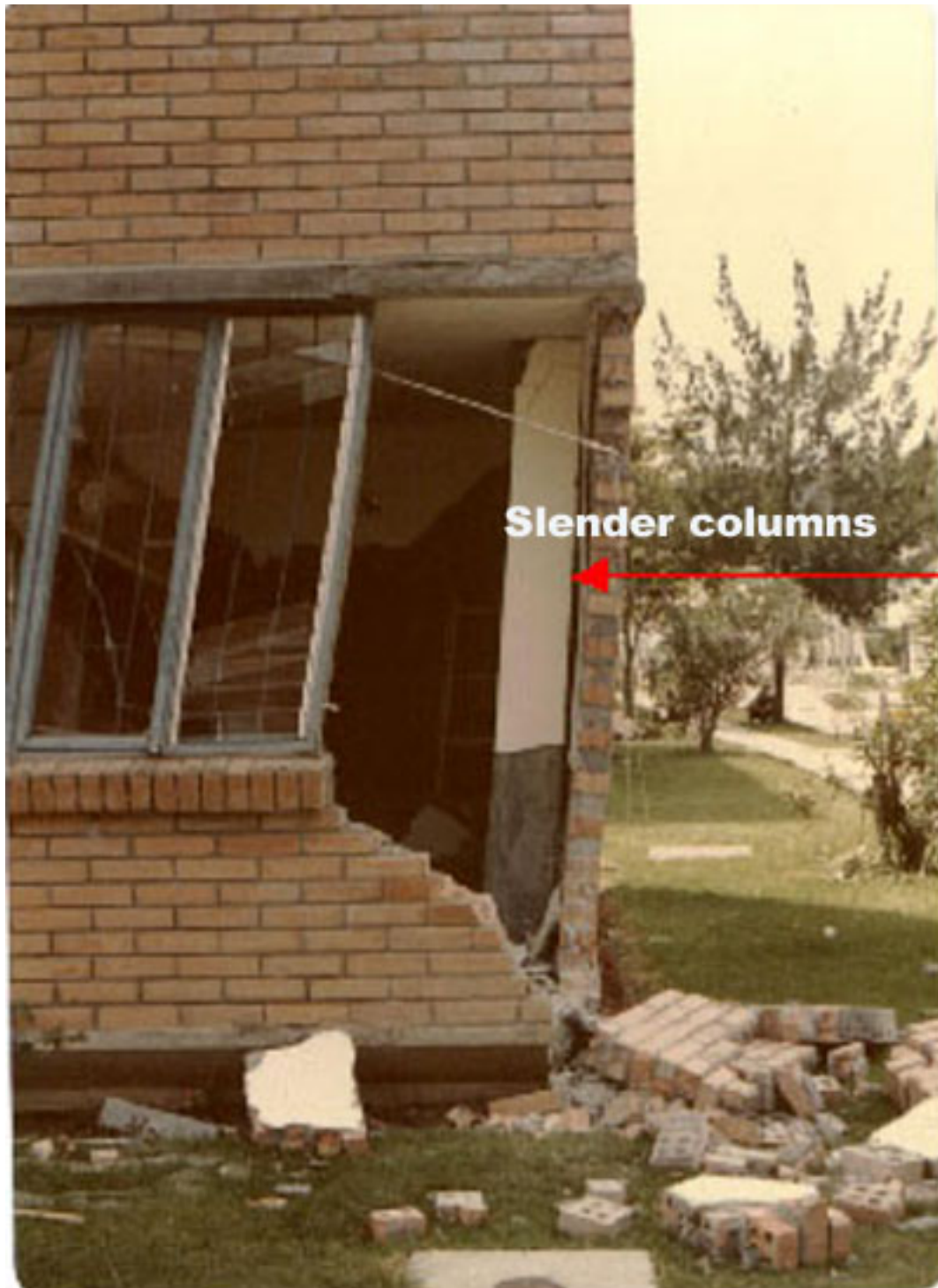
FIGURE 6I: Earthquake Damage- Very Slender Columns
