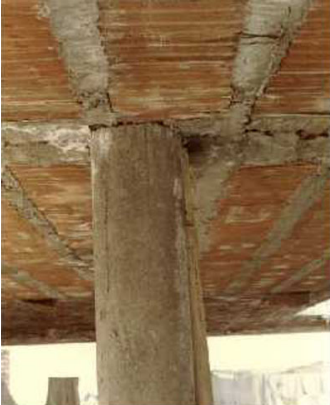
FIGURE 5I: Poor Construction Practice-Drains running across the girders. Stirrups are removed to allow for the pipeline passage
