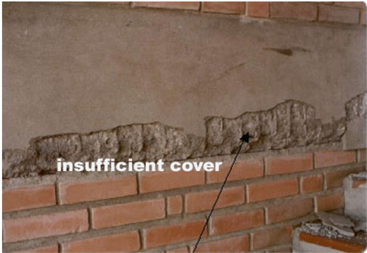
FIGURE 6K: Earthquake Damage-Inadequate Concrete Cover
