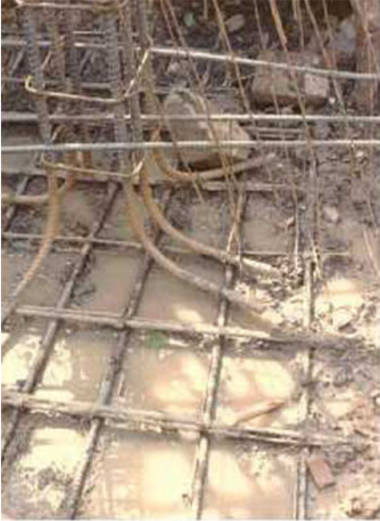
FIGURE 5H: Poor Workmanship - Dirty groundwork and inappropriate column and bar anchorage
