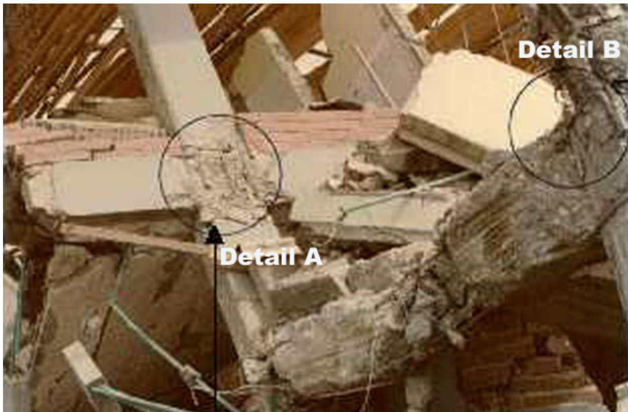
FIGURE 6B: Earthquake Damage- Reinforcement splices in the joint zone (Detail A).
