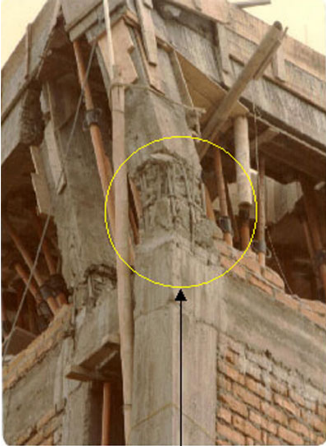
FIGURE 6J: Earthquake Damage-Inadequate Column Splices
